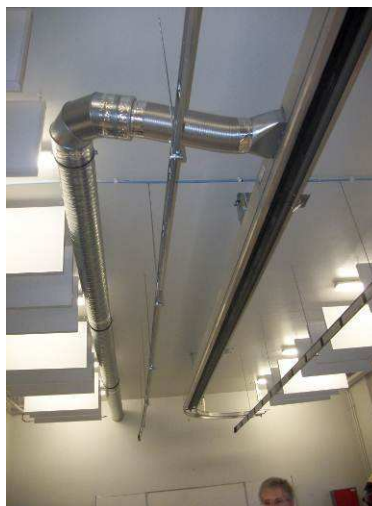
Rail et gaine d'évacuation Atelier C003
